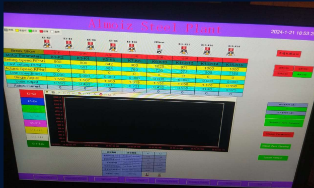
SCADA System (Operating Room)
